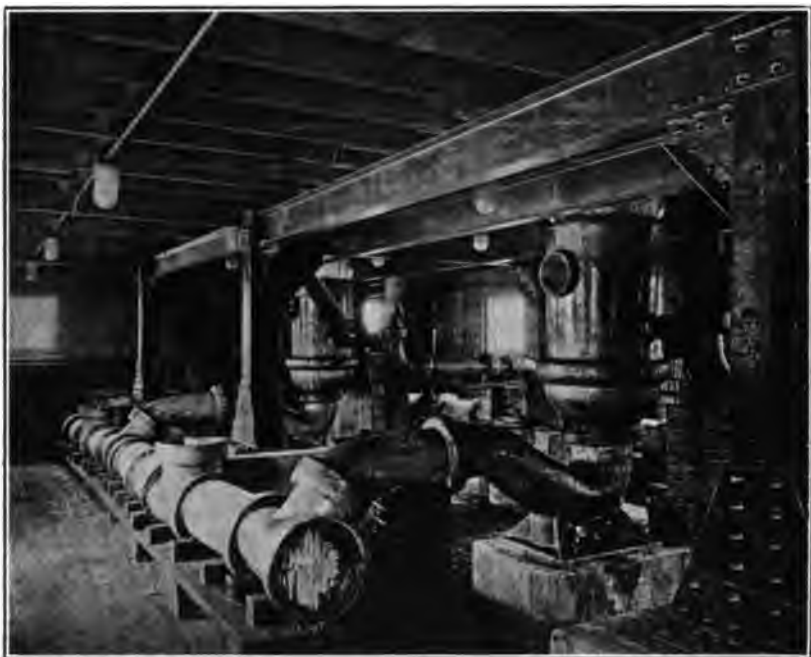
PLATE 3.—DU PONT MECHANICAL DIFFER PROCESS, IMMERSING BASIN AND EXIT FLUME FLOOR, SMOKELESS POWDER FACTORY, PICATINNY ARSENAL, N. J.
